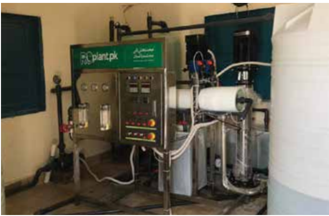
An RO plant at Moriro Markaz.
