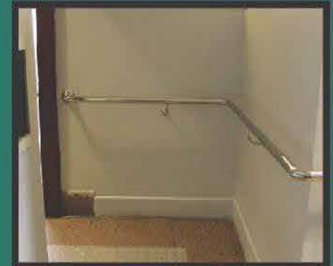
Handrails to encourage easy maneuvering for persons with disabilities within the office space
