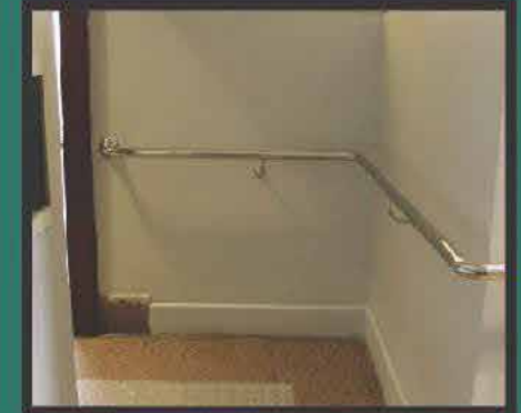
Handrails to encourage easy maneuvering for persons with disabilities within the office space
