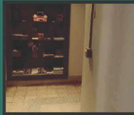
Height adjusted switchboards and door handles for persons with physical impairments
